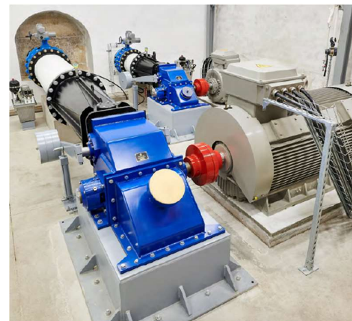
Turbines Crossflow, centrale de Consolation (25).
